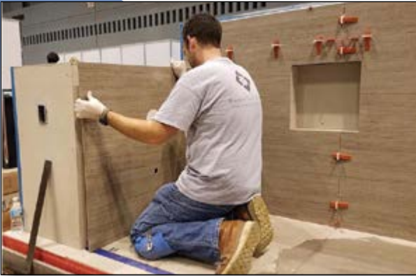
Dean Gottschalk from Bourbon Tile & Marble performing the ACT Thin Porcelain Tile test at the 2016 Covering show.
